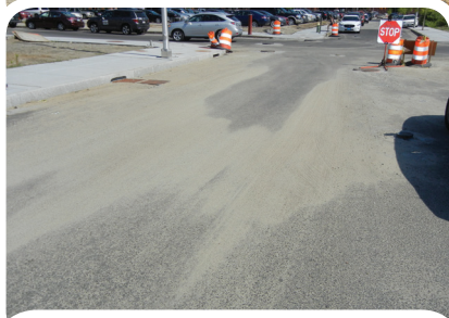
The sediment in this roadway is a public safety hazard.
