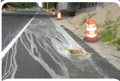
Concrete outwash, which is highly toxic to aquatic life, was being carried by runoff to a storm drain.
