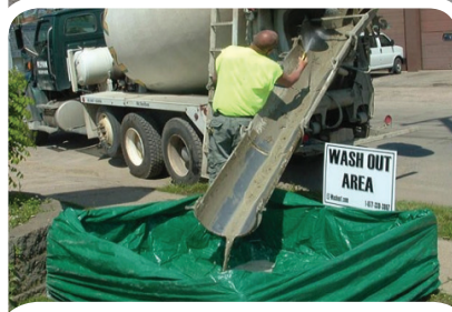
The use of a concrete wash out area allows for containment of water that is generated from washing out ready-mix equipment.
