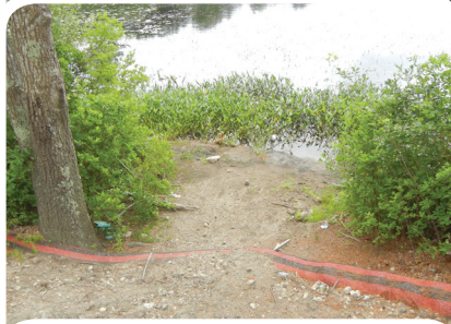
Sediment trapped on the construction side of compost filter socks must be collected and removed regularly.
