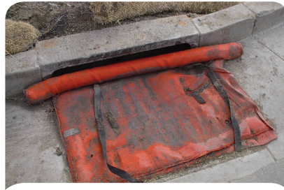
Filter fabrics on storm drains are a last line of defense against sediment entering waterways. Photo credit: US EPA.
