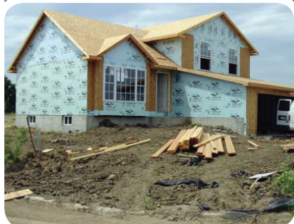
A small construction site with no visible erosion control measures. Photo credit: iowastormwater.org .
