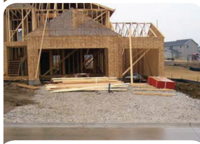
Crushed stone has been placed at the construction site access, which reduces sediment being tracked into roadways. Photo credit: iowastormwater.org .
