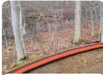
This filter sock is appropriately placed between construction and a wetland. The area is free of accumulated sediment.
