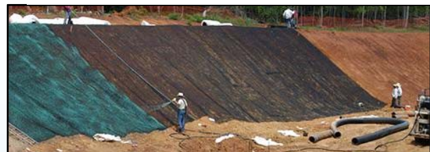
Turf reinforcement matting used on a slope to help hydroseed adhere and prevent erosion
