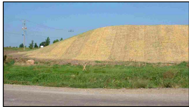
Straw blankets applied to a stockpile to prevent erosion and sedimentation during a shut-down period
