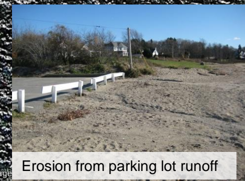
Erosion of western parking area
