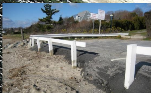
Before: Erosion of western parking area
