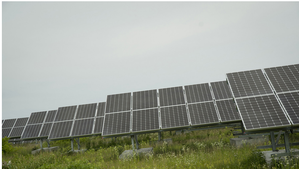
The solar panel field in West Kingston is located on a capped waste disposal site. It was developed and is owned by Kearsarge Energy as part of the URI-led South Kingstown Solar Consortium, which includes the towns of Narragansett and South Kingstown. (URI photo/Nora Lewis)
