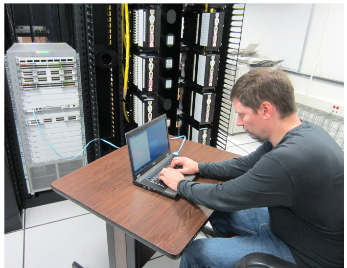
Mark Fester, ITS network technician, configures a Cisco Nexus switch in Tyler Hall's data center, part of the new fiber optic data network. Photo by: Mike Stewart/ITS
