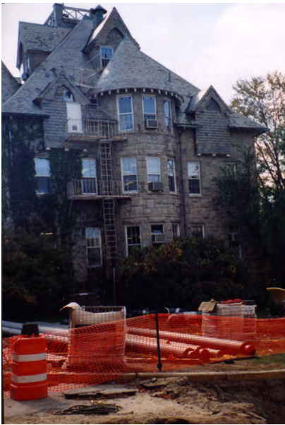
The University is now addressing years of deferred maintenance, allowing it to move forward unencumbered in the next century.
