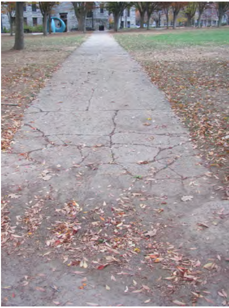
Walkway in poor condition
