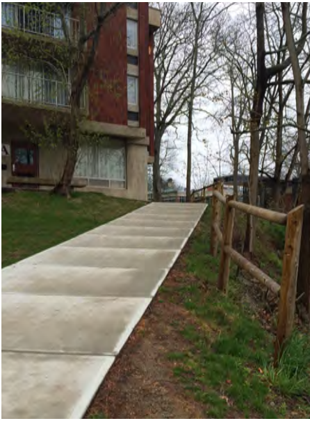
Lack of appropriate handrail
