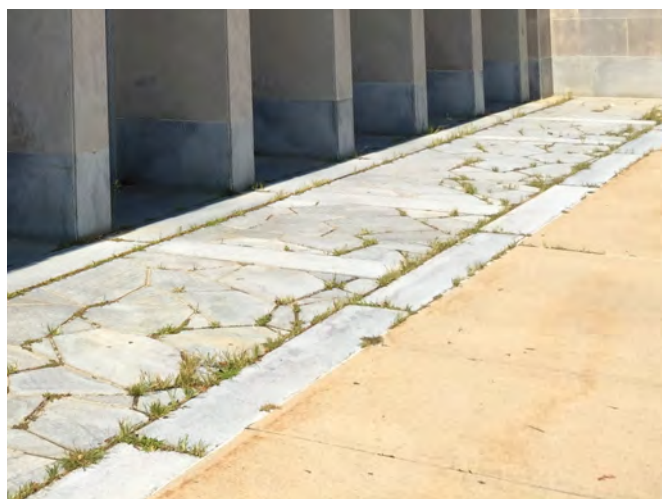
Hardscape material should be selected based on the ability to maintain it. Joints in this irregular flagstone require routine maintenance and removal of weeds with herbicide.
