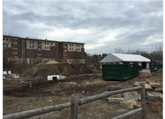
Storage facilities should be improved to safely store equipment and materials.
