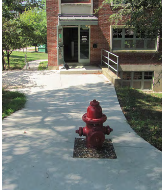
Obstructions within hardscapes can be accidentally hit during snow removal.
