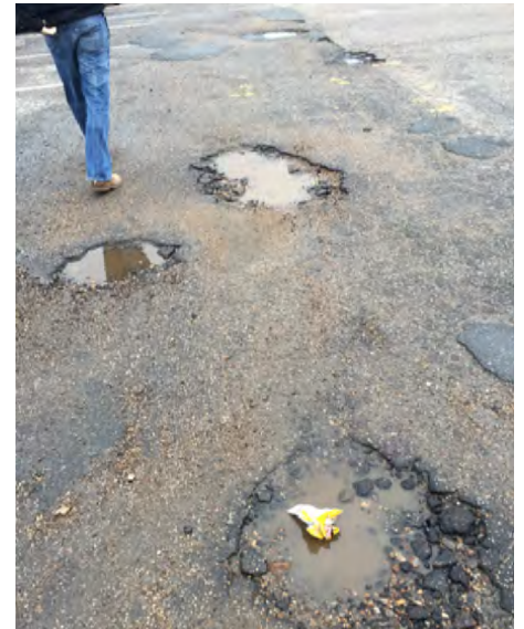
Excessive potholes in parking lots
