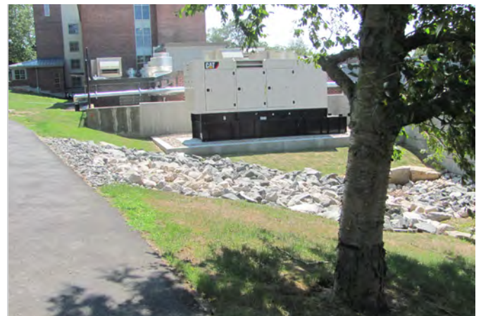
Riprap was added to a sloped swale to reduce erosion and improve drainage, however this is not the most visually appealing solution.
