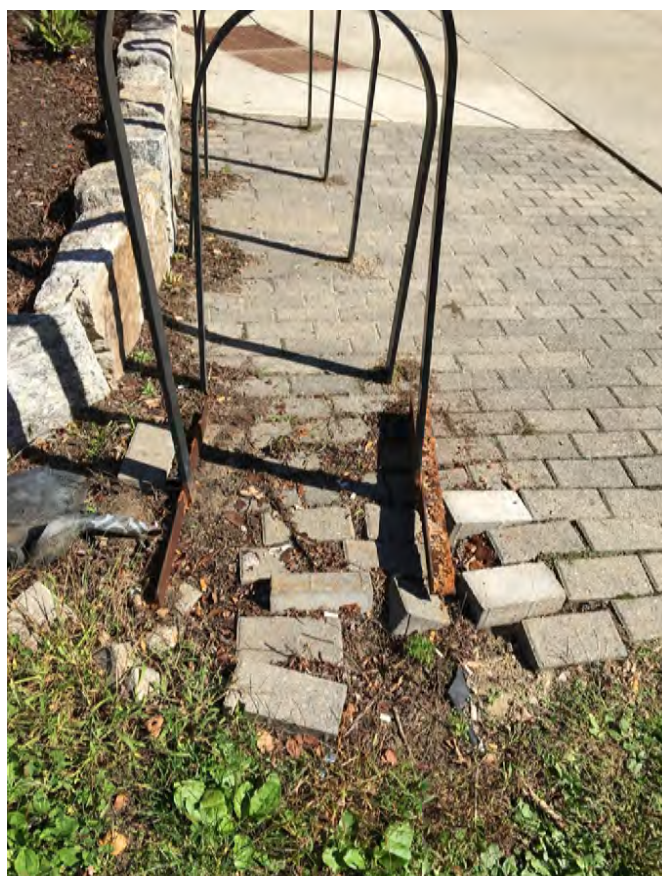
This bike rack was likely damaged by an careless use of machinery.
