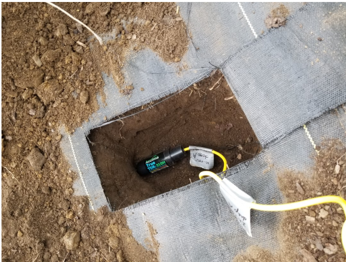
A sensor inserted sideways at 8" deep.
