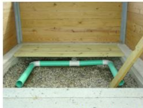
Forced aeration. A powered blower will force air through this pipe to the compost pile. A slotted wooden floor will cover the aeration pipe.
