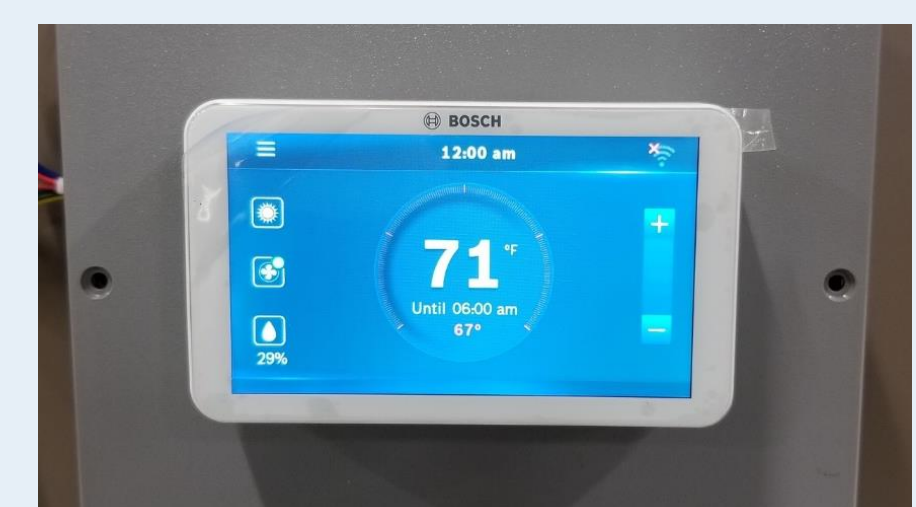
Figure 3 – Control Housing with Bosch Connected Control Thermostat
