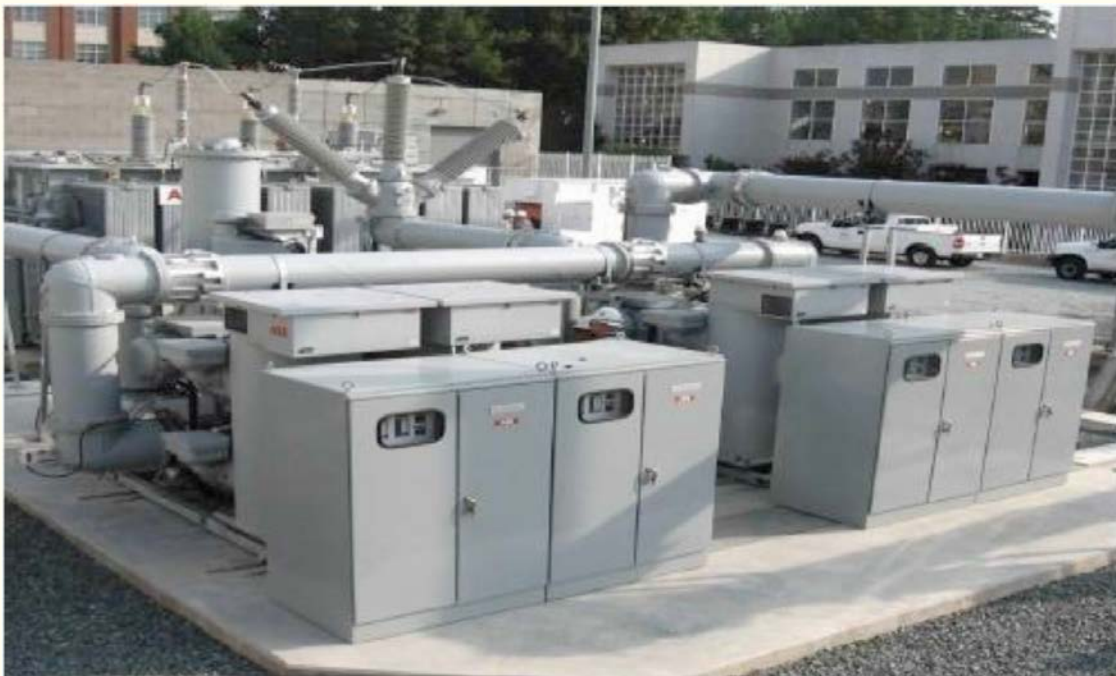
Fig 1: Local control cabinet and high voltage equipment
