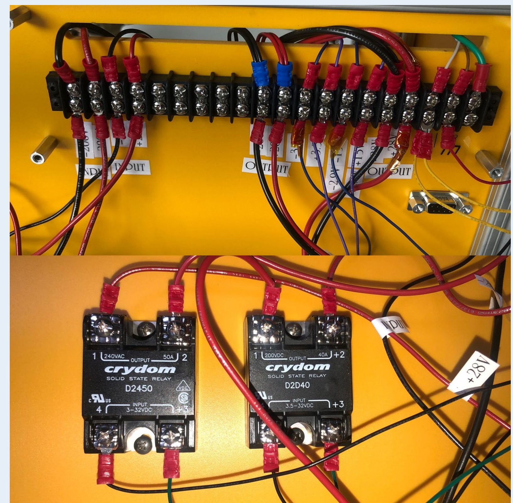
Fig.2: Wiring on DUT Enclosure
