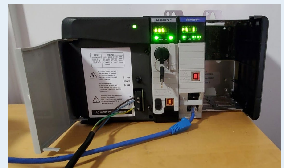
Fig. 2 - Programmable Logic Controller with, from left to right, the Processor and the Ethernet card.
