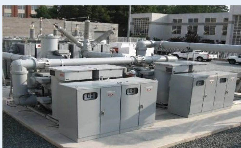
Figure 4: Local Control Cabinet and High Voltage Equipment
