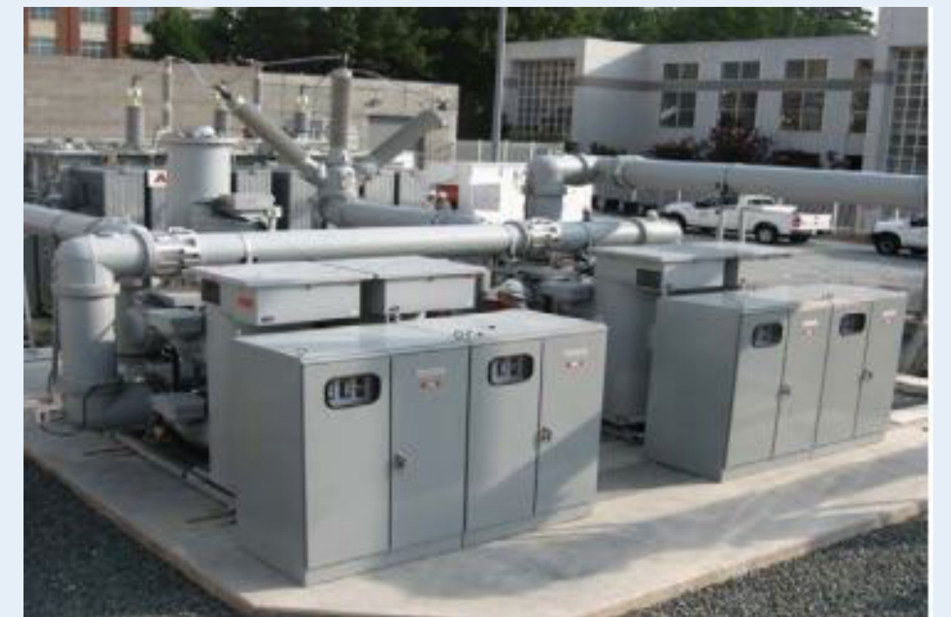
Figure 1: Local Control Cabinet and High Voltage Equipment field installation
