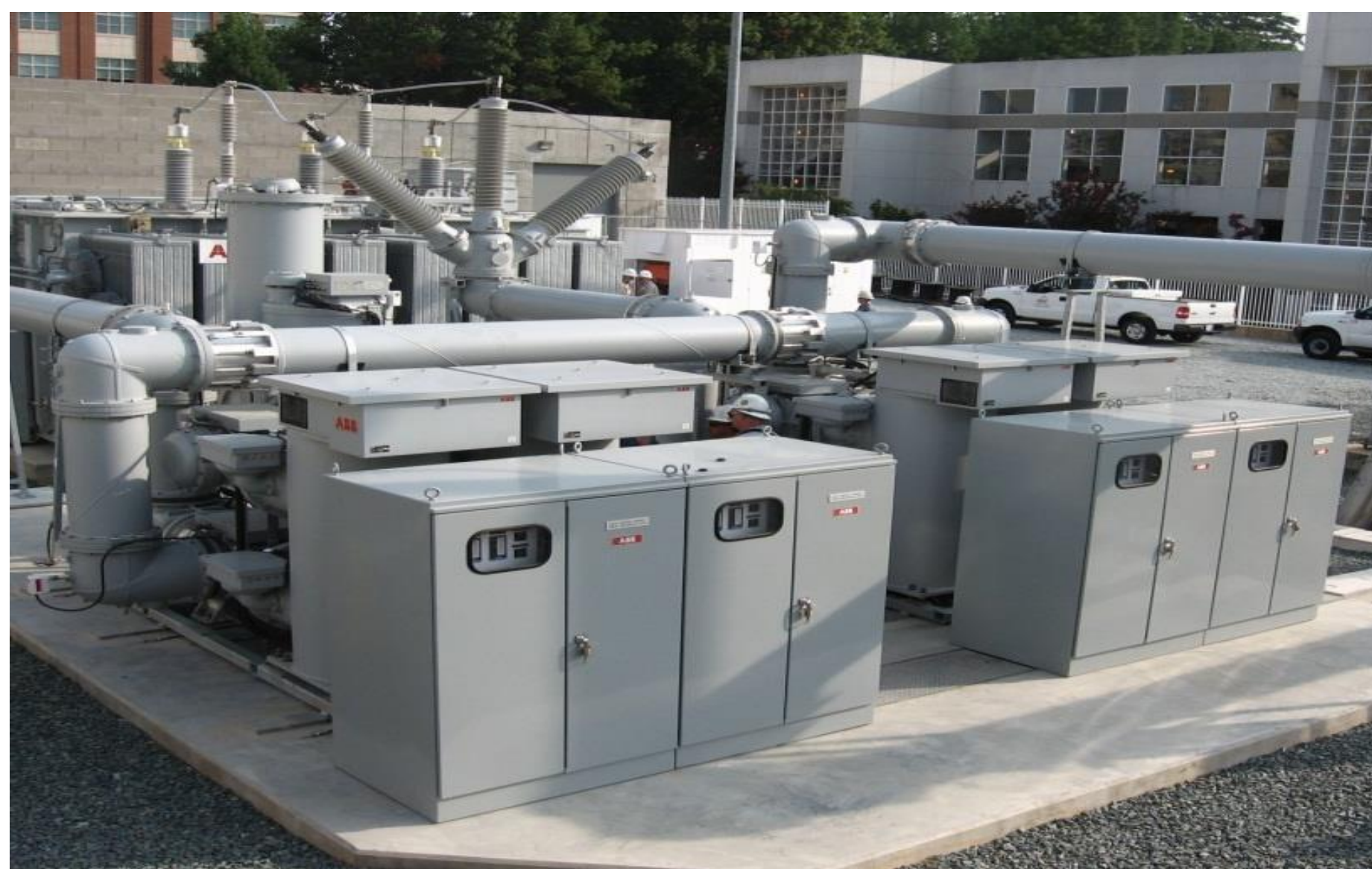
Typical Gas Insulated Substation
